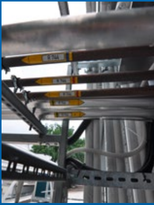
▲ The CO 2 cycle operates exclusively between the technology room and components installed outdoors such as the Güntner gas cooler.
