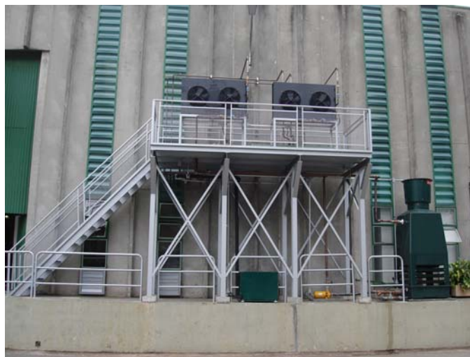
Figure 08: Detail of the air-cooled condensers and the water-cooling tower.
