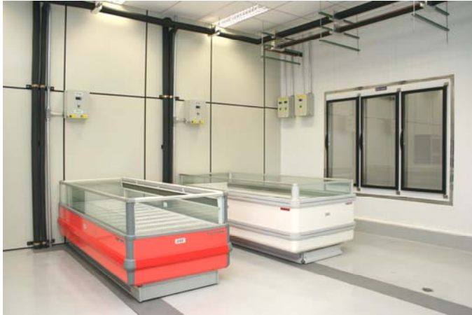
Figure 02: Detail of the islands and walk-in cooler.
