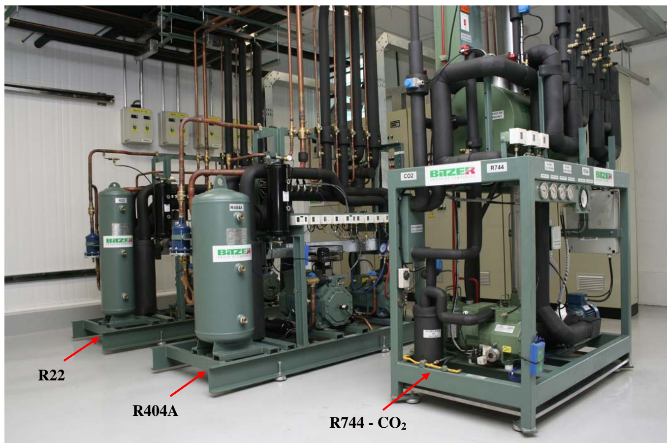
Figure 01: Detail of the refrigeration racks from the CO 2 Technology & Training Center of Bitzer Brazil.
