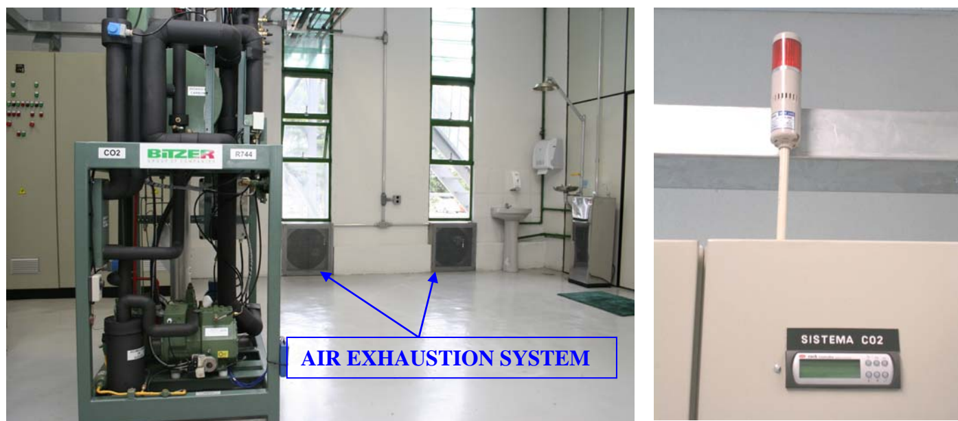
Figure 15: Detail of the air exhaustion system and the alarm system in the case of any CO 2 leak.
