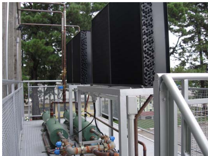
Figure 07: Detail of both the air and water-cooled condensers.
