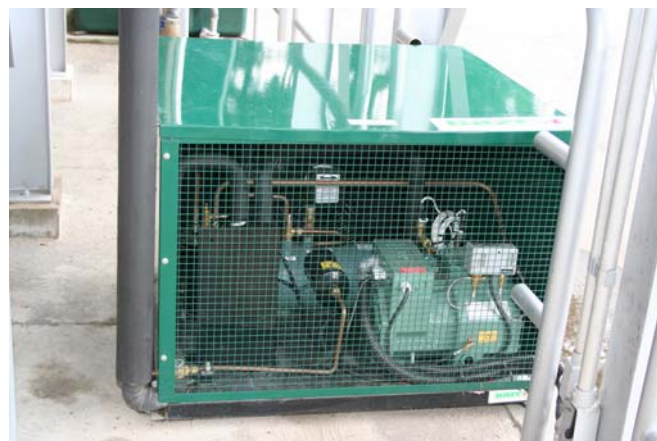
Figure 16: CO 2 standby system.
