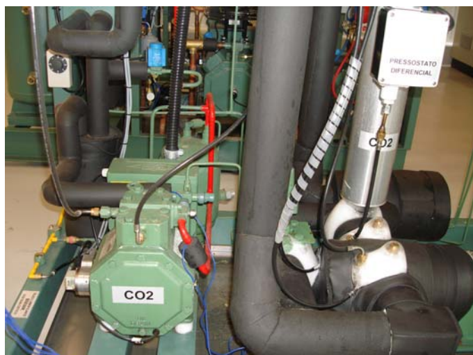
Figure 05: Detail of the CO 2 compressor.
