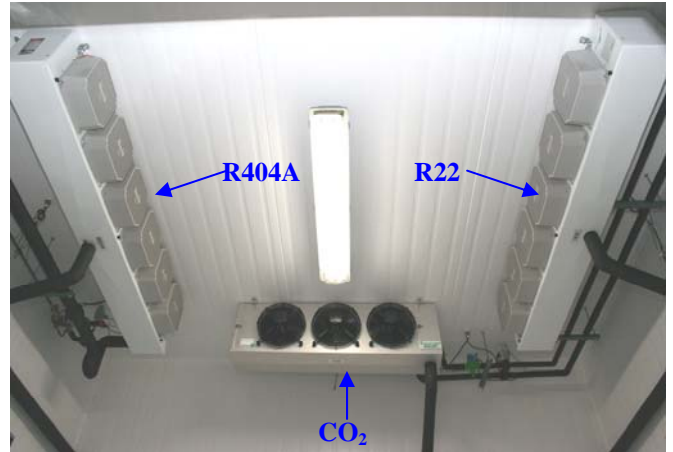
Figure 03: Detail of the air coolers installed in the cold rooms for medium and low temperature.
