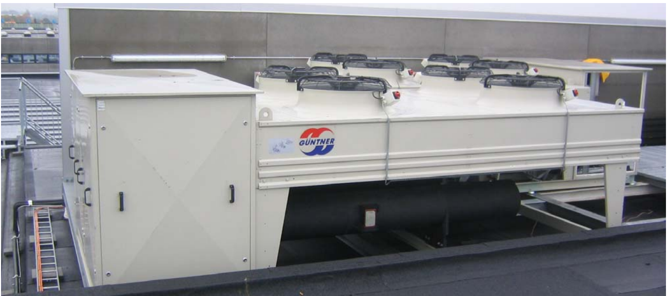
Figure 7: 2 prototype units installed 2004 at the roof of a shopping Centre in Copenhagen.
